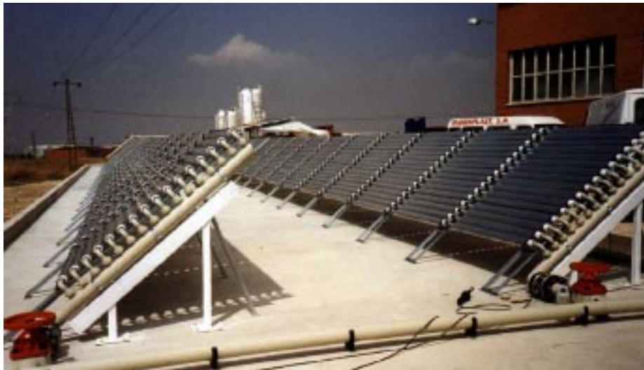
Fig. 1. View of a SOLARDETOX treatment plant installed at Hidrocen factory (Madrid, Spain)
